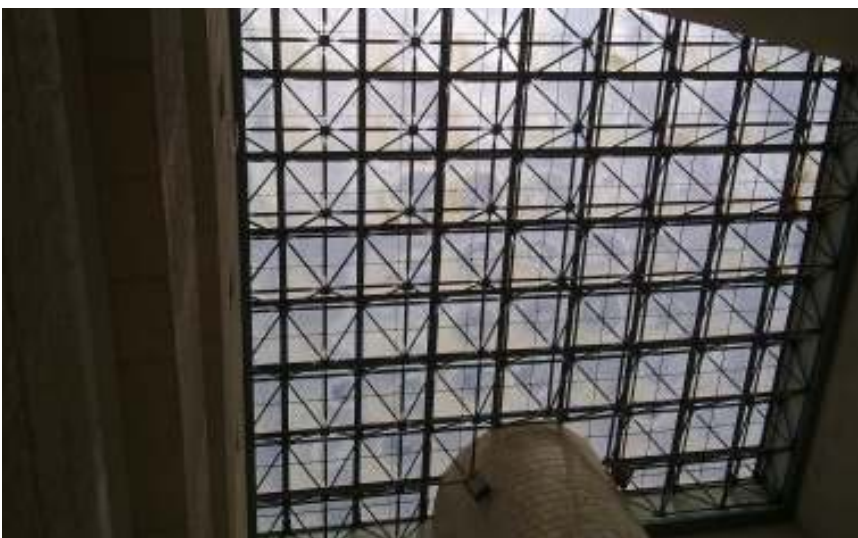
Figure (34): School of Fine Arts at An-Najah National University (A view showing the court yard roof) Photo by: the author, 2011.
