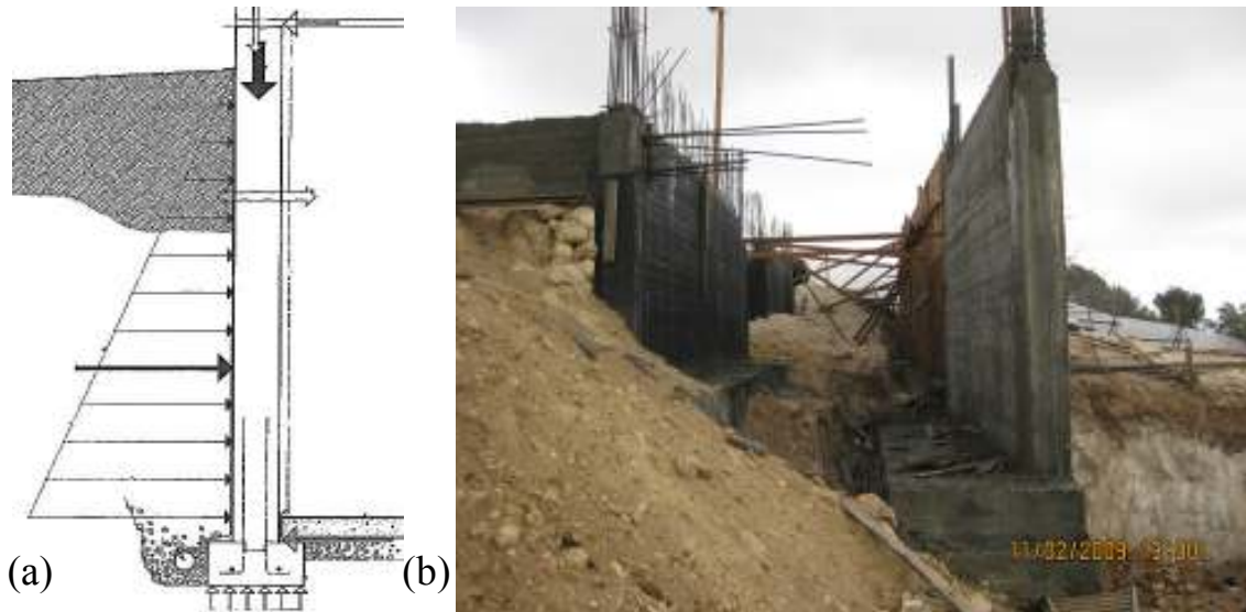
Figure (16): (a) A section in a Foundation Wall, (b) Photo of a foundation wall in a project in the West Bank
